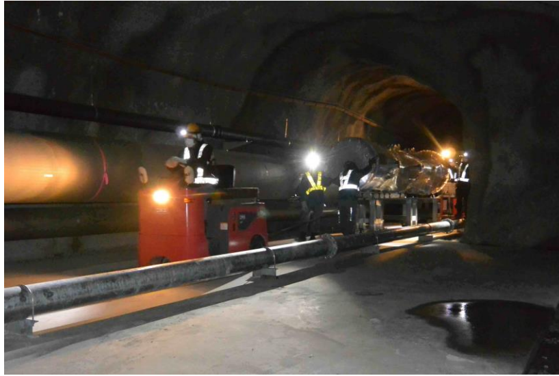
X-end cryostat assembly
